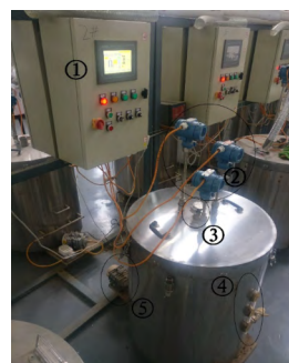
①通风、温度控制系统 ②温度采集器 ③气体采样孔 ④固体采样孔 ⑤气泵 ①Ventilation and temperature control system ②Temperature collector ③Gas sampling hole ④Solid sampling hole ⑤Air pump
